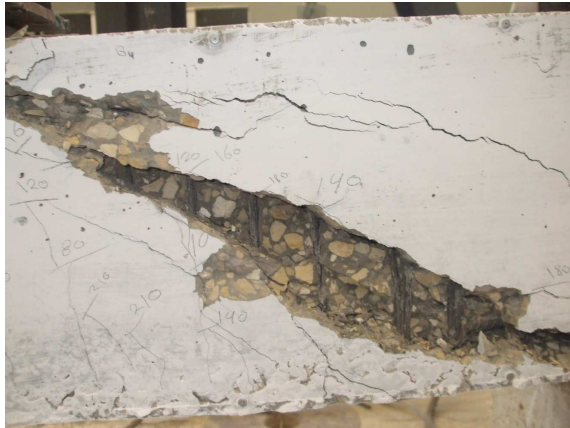
Figure 3: Beam B4 mode of failure at 230 kN applied load.
